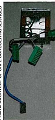
An Edge pre-wiring with reader, REX, lock and network connections.
